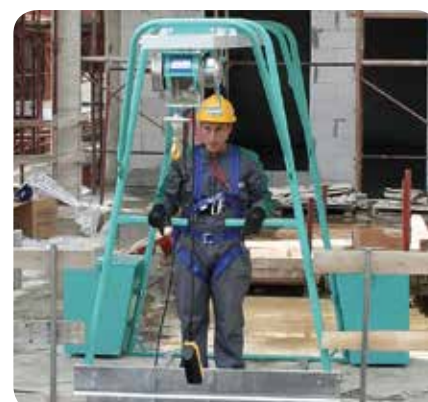
Gantry for stand hoists
