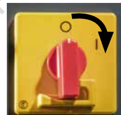
Switching on the main switch
